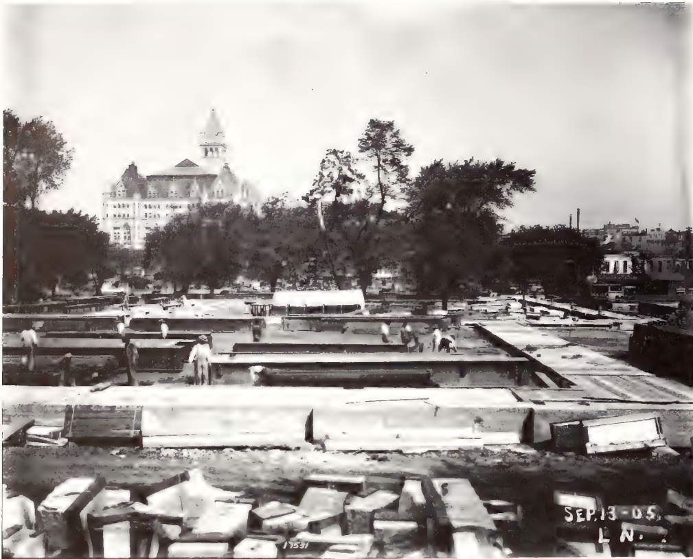
Construction on the ground floor at the west side of the building, looking north toward the Post Office. September 13, 1905.
